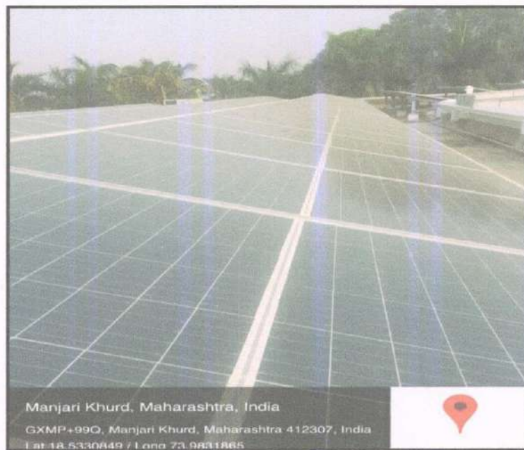
Photograph of Roof Top Solar PV Plant:
